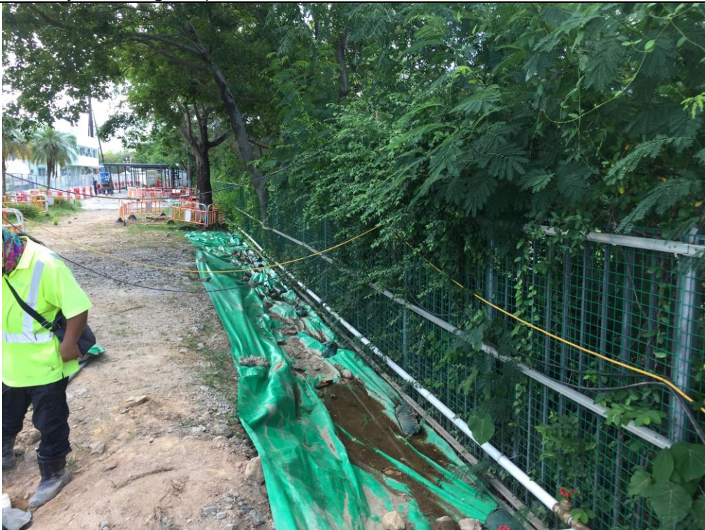
Date of site inspection: 15 July 2021 The surrounding of the construction site areas were covered by impermeable sheeting to prevent surface runoff.
