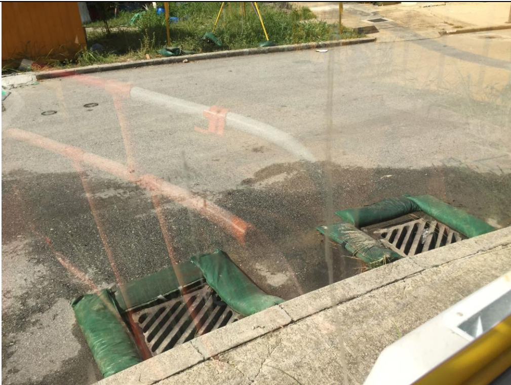
Date of site inspection: 15 July 2021 Gullies were banded by sand bags to prevent surface runoff.
